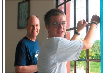
Duncan and Charlie Healy working on the front doors of the church.
